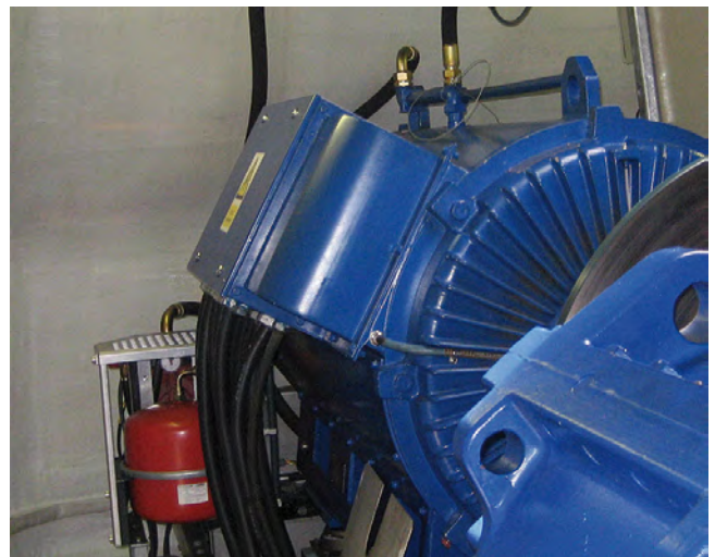
Generator in a wind turbine
